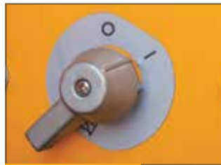
BATTERY DISCONNECT SWITCH
